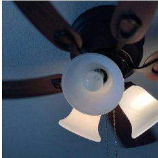
Light Fixture / Fan (1/2) 05/24/2021 12:24 PM
