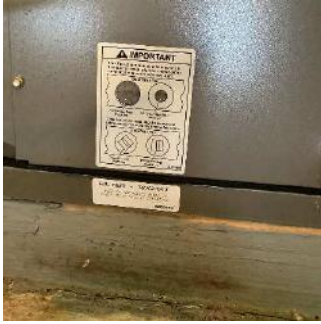
HVAC Return / Filter (Location and Size) (3/4) 05/24/2021 12:28 PM
