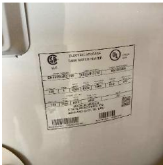
Water Heater (3/3) 05/24/2021 12:12 PM
