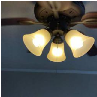
Light Fixture / Fan 05/24/2021 12:25 PM
