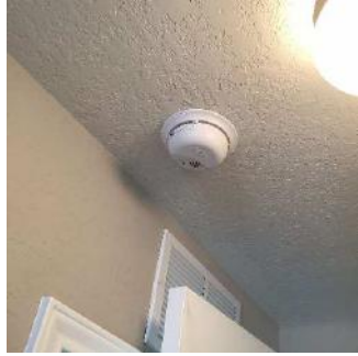
Smoke Alarm 05/24/2021 12:26 PM
