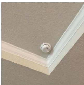
Smoke Alarm 05/24/2021 11:53 AM
