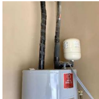
Water Heater (1/3) 05/24/2021 12:12 PM
