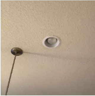
Light Fixture / Fan 05/24/2021 11:58 AM
