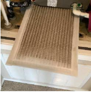
HVAC Return / Filter (Location and Size) (2/4) 05/24/2021 12:27 PM
