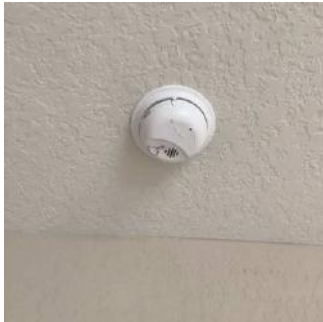
Smoke Alarm 05/24/2021 12:25 PM
