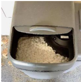
Water Softener / Salt Levels (2/2) 05/24/2021 12:12 PM
