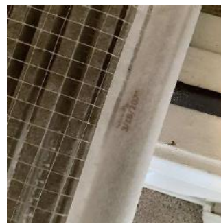
HVAC Return / Filter (Location and Size) (1/4) 05/24/2021 12:27 PM
