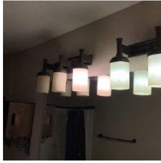
Light Fixture / Fan 05/24/2021 12:37 PM
