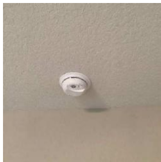
Smoke Alarm 05/24/2021 12:32 PM
