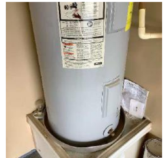
Water Heater (2/3) 05/24/2021 12:12 PM
