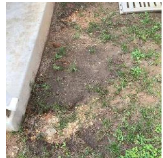
Signs of Erosion/Drainage (2/2) 05/24/2021 11:35 AM
