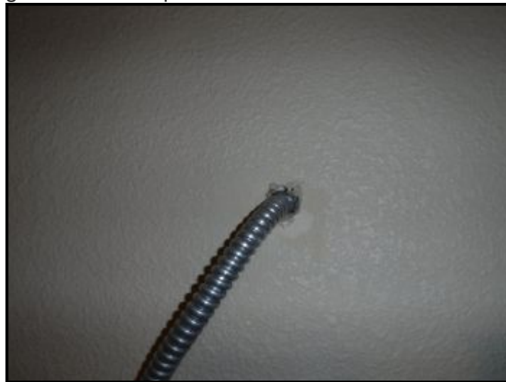
Recommend caulking around conduit
