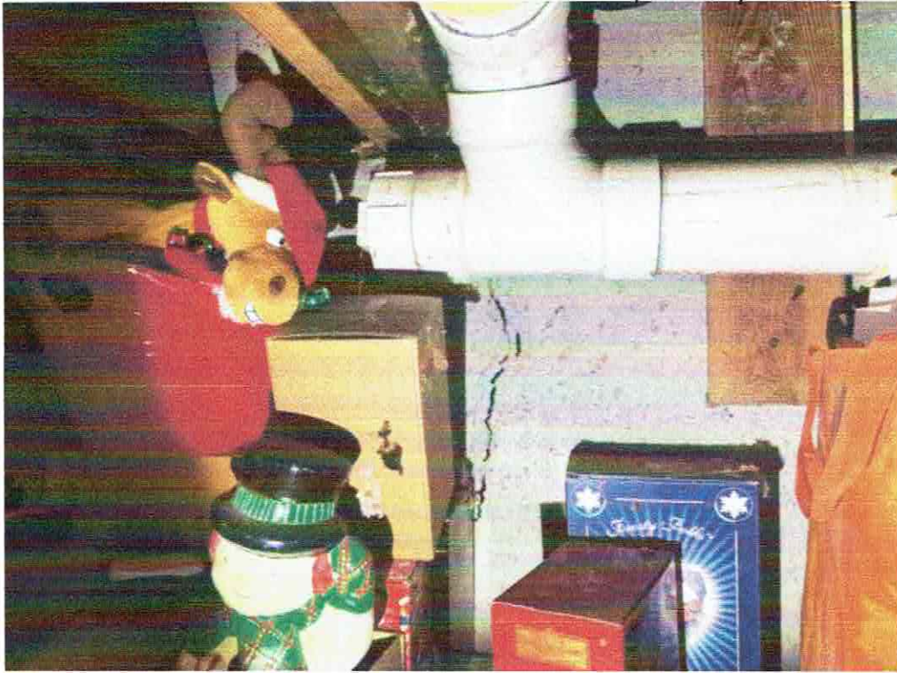
View of crack in left wall of foundation seen from basement.
