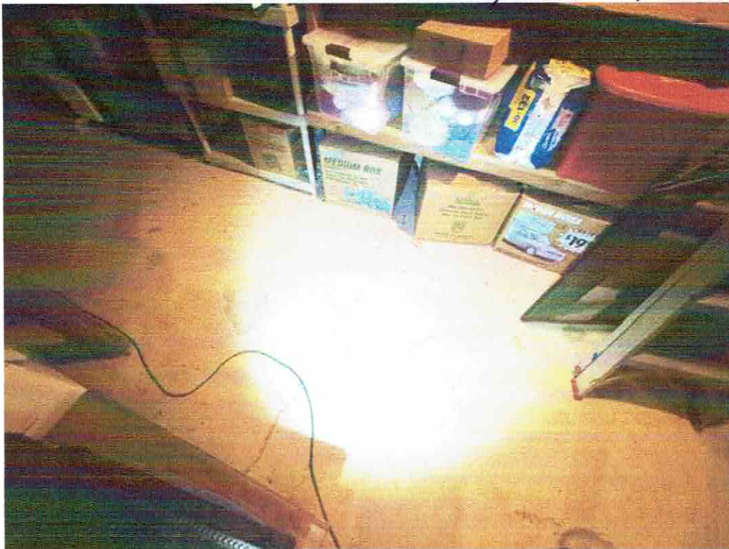
View of cracks in basement floor slab.
