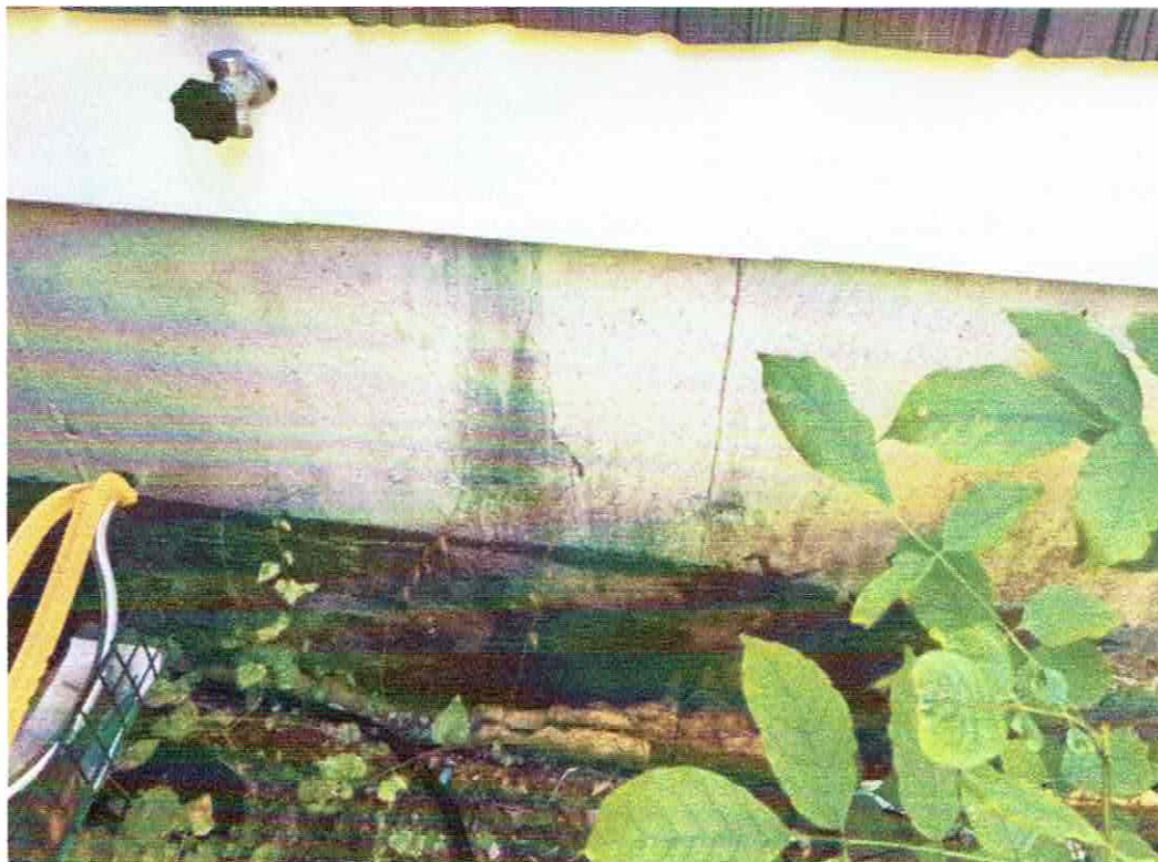
View of settlement crack in rear wall near left corner of house foundation.
