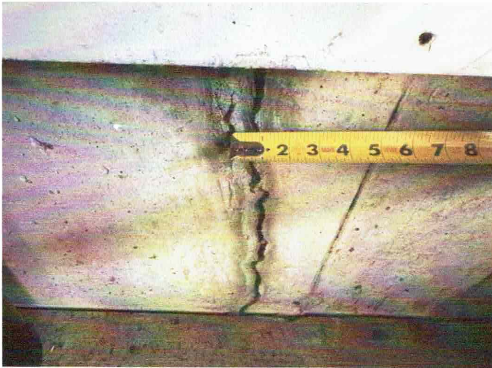
View of crack in left wall of house foundation.
